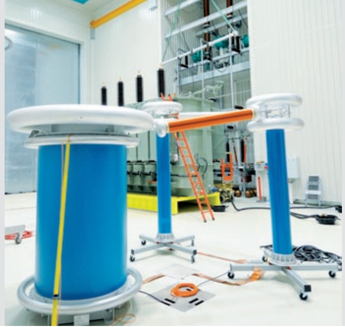
Fig. 2 Applied voltage test system for testing of power transformers, type WRV 5/360 M
