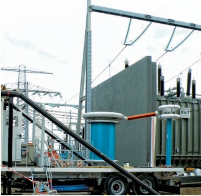
Fig. 1 Applied voltage test system for on-site testing of power transformers, type WRV 5/360 M
